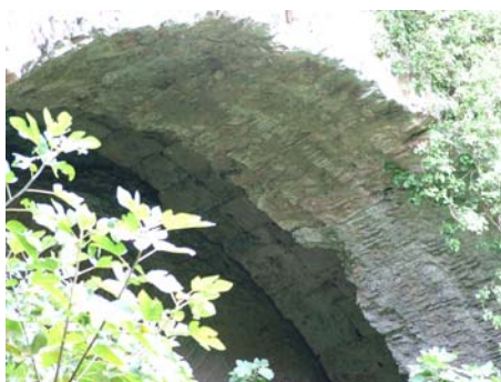
Figure 4 : Strengthening work of St. Peter's bridge: multi-ring arch framework in opus caementicium . See also, in the middle between the new arches, the old stone arch in square blocks
